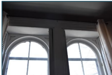
Figure 56: Cracking in window framing
