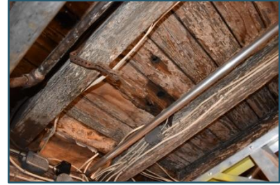
Figure 93: Moisture staining in ceiling framing
