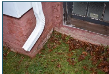
Figure 11: Ground underneath downspout sunk around building
