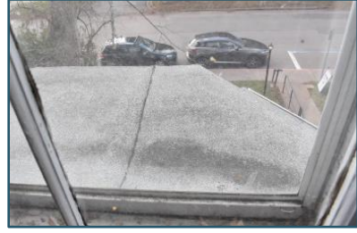
Figure 39: Moisture accumulation on lower roof
