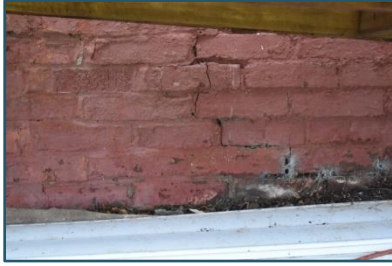
Figure 79: Cracking in east foundation
