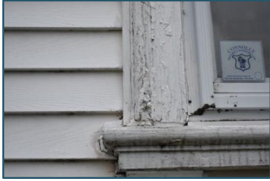
Figure 20: Deterioration of wooden window frame
