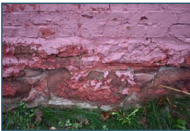
Figure 76: Deteriorating stone on east facade
