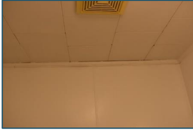
Figure 61: Poor seals at joint between walls and ceiling in bathrooms
