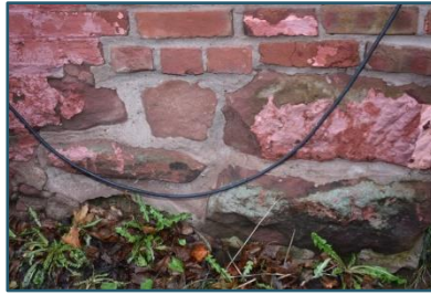
Figure 83: Thick joints in repair mortar
