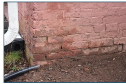
Figure 75: Open joints in masonry on front facade
