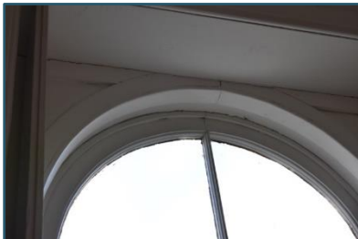
Figure 55: Cracking in window framing
