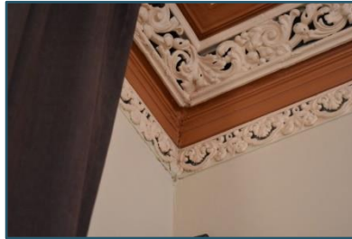
Figure 50: Crack in corner cornice detail
