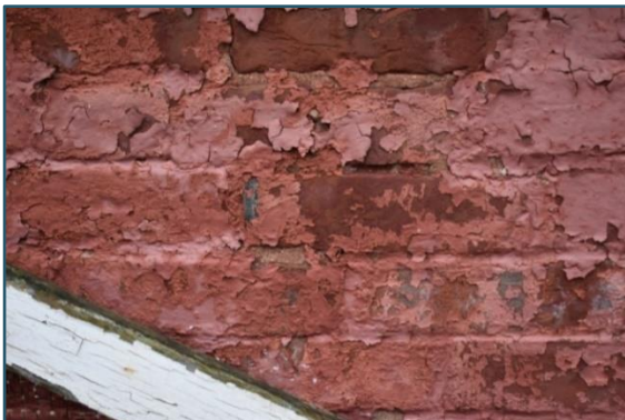
Figure 112: Incompatible paint on brick
