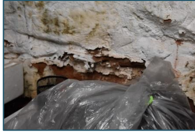
Figure 92: Failing paint from high moisture content in walls
