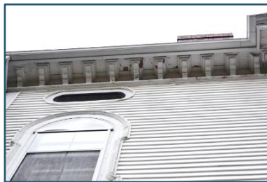
Figure 18: Failed paint at the decorative brackets
