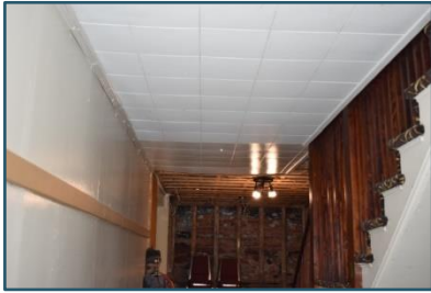
Figure 94: Deflecting ceiling tiles
