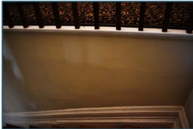
Figure 52: Plaster cracking in staircase
