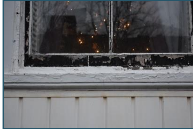
Figure 21: Deteriorating window sash
