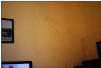
Figure 67: Plaster cracking in Club Manager's Office
