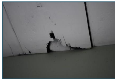
Figure 26: Broken ceiling board
