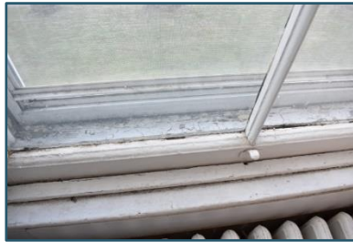
Figure 65: Paint failing around window
