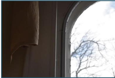
Figure 49: Poor seal around window in sitting room
