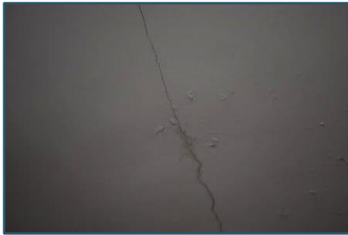
Figure 64: Staining around crack in ceiling
