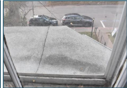
Figure 108: Roof staining indicating an area prone to water accumulation
