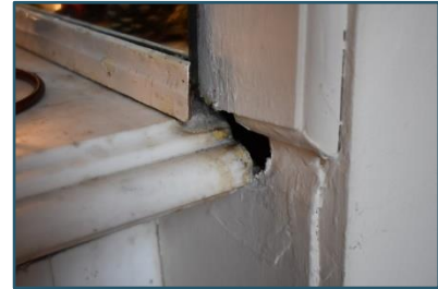
Figure 51: Gap between chimney mantel and wall
