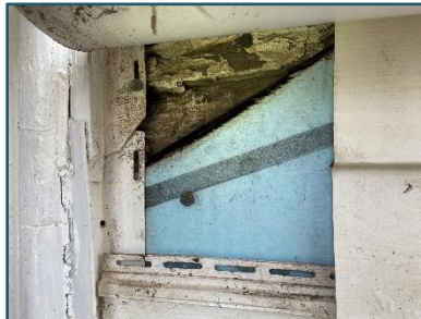
Figure 24: Damaged clapboard siding covered by vinyl siding, photo provided by Greg Munn on 2022-12-20
