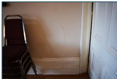
Figure 41: Plaster crack in main room
