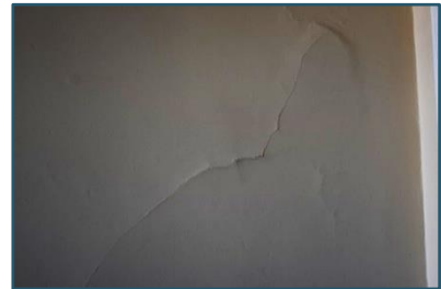
Figure 69: Plaster cracking in dressing room
