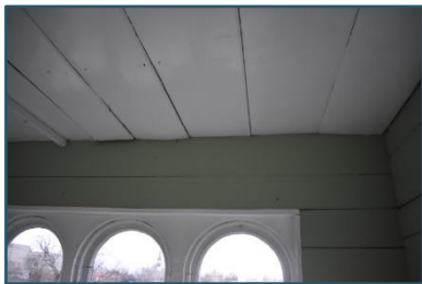
Figure 25: Uneven ceiling boards in belvedere
