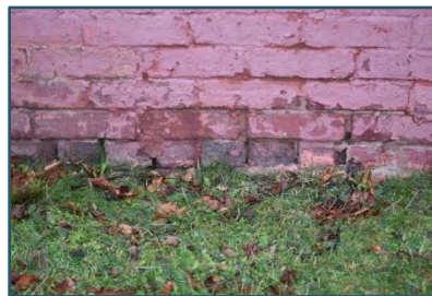
Figure 74: Open joints in brick at base of wall on south facade
