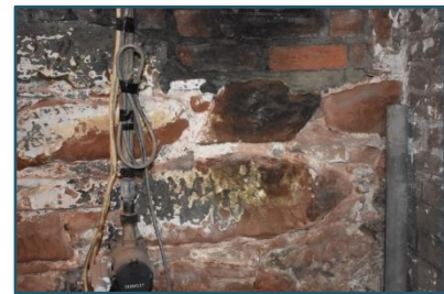
Figure 102: Failing paint on masonry
