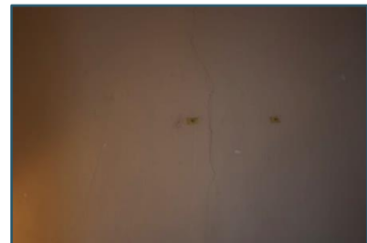
Figure 42: Plaster crack in main room
