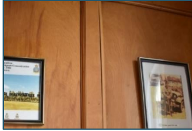
Figure 62: Wood panelling becoming detached
