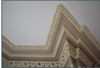
Figure 47: Damaged and repaired cornices
