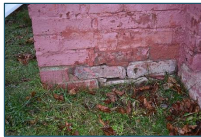
Figure 77: Deteriorating stone on south facade
