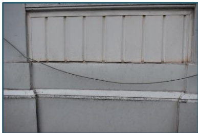
Figure 14: Opening in junction between siding
