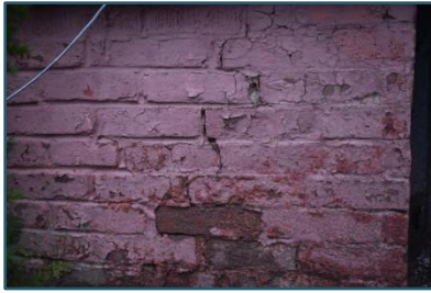
Figure 82: Cracking in foundation at southwest corner
