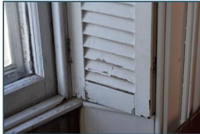
Figure 53: Failing paint on window shutters
