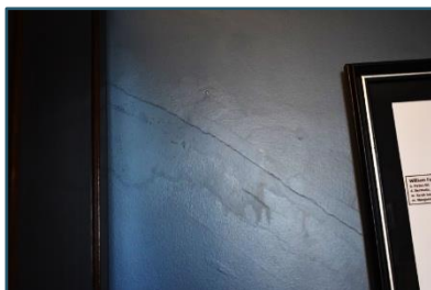
Figure 70: Plaster cracking in Captain's room
