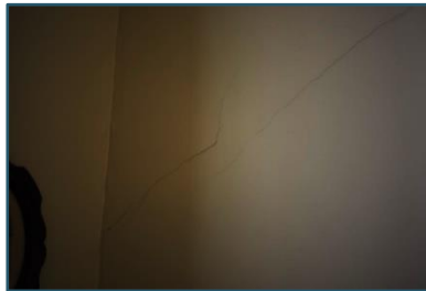
Figure 68: Plaster cracking in dressing room
