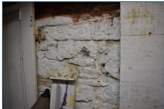
Figure 113: Incompatible paint on interior foundation masonry
