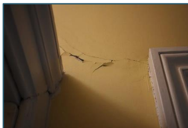
Figure 71: Plaster cracking at storage area south of bathrooms
