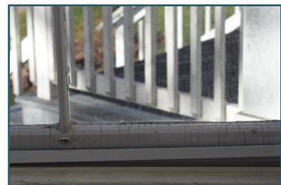
Figure 45: Failing window paint
