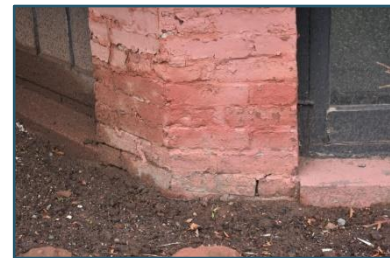
Figure 12: Window wells set too close to ground
