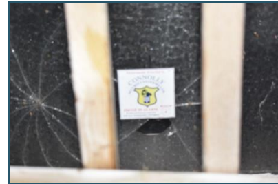
Figure 84: Broken window well
