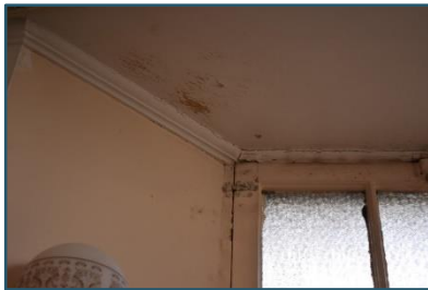
Figure 85: High moisture content around front facade window wells
