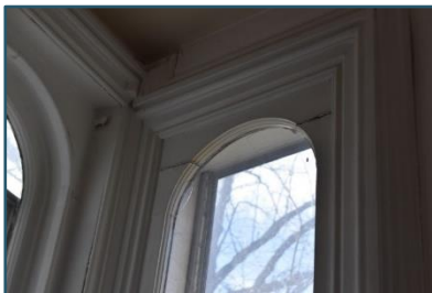
Figure 40: Horizontal cracking in window frame at vestibule
