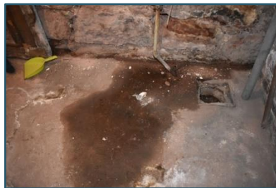
Figure 101: Moisture around leaking pipe
