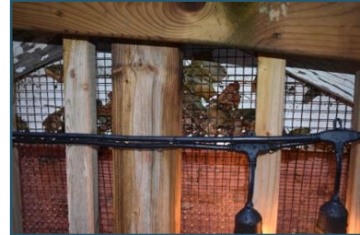
Figure 22: Ramp railing trapped debris towards the building
