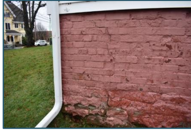
Figure 80: Cracking in foundation at southeast corner
