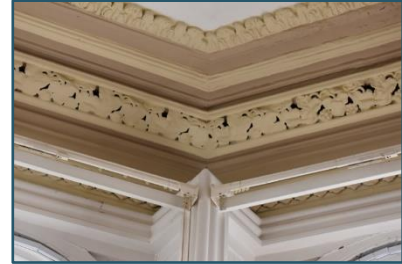
Figure 48: Change in detail where cornice was damaged
