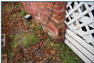
Figure 10: Ground immediately adjacent does not slope away from building
