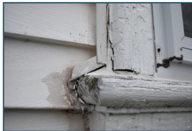
Figure 15: Worn joint between siding and wooden windowsill
