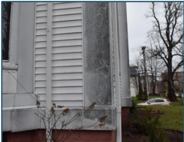
Figure 23: Surface staining at southwest corner
