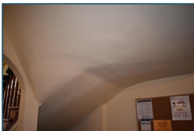
Figure 43: Plaster cracking underneath main staircase
