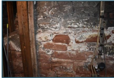
Figure 98: Damaged foundation masonry
