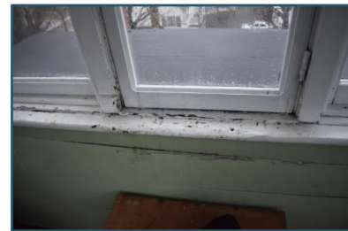
Figure 27: Condensation on windows and high moisture content in walls
