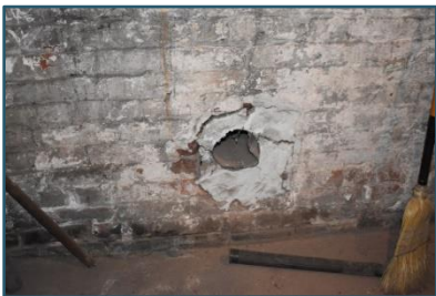
Figure 100: Masonry damaged around utility opening
